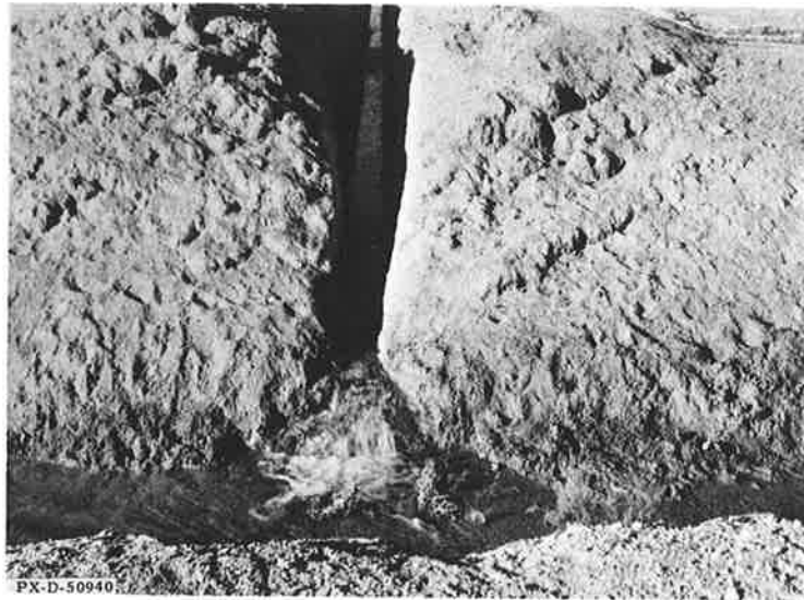
Figure 18. --Most farmers in the Valley were aware of the need and usefulness of farm drains. Drains such as this one dug by hand furnish much needed employment for farmers during seasons of slack farmwork.
