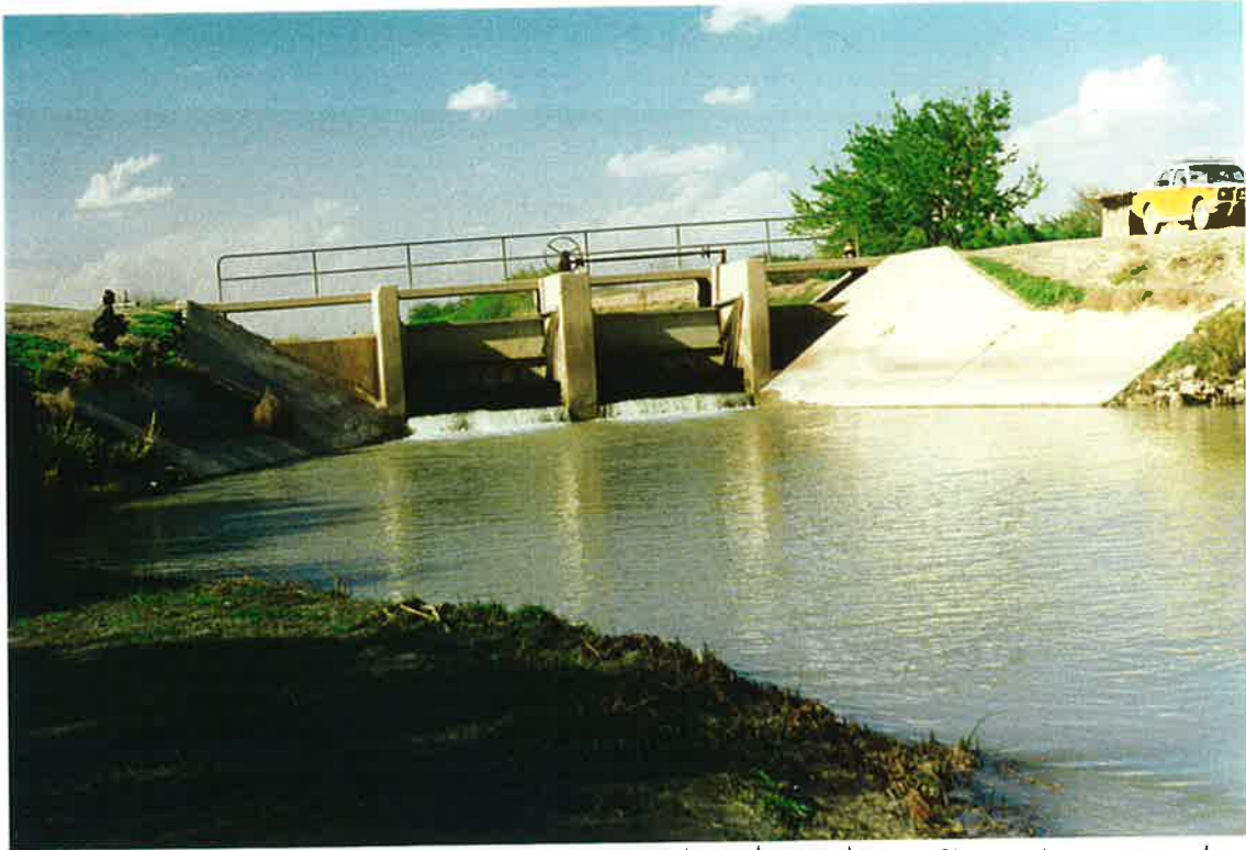
33. Diversion structure for S-10,7 lateral on the Shamalan canal. Gates closed. Lift mechanism not functioning. 21 March 97
