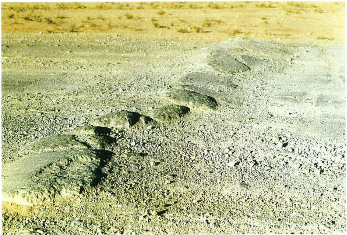
8. Kandahar to Herat highway broken road surface 20 Oct 97
