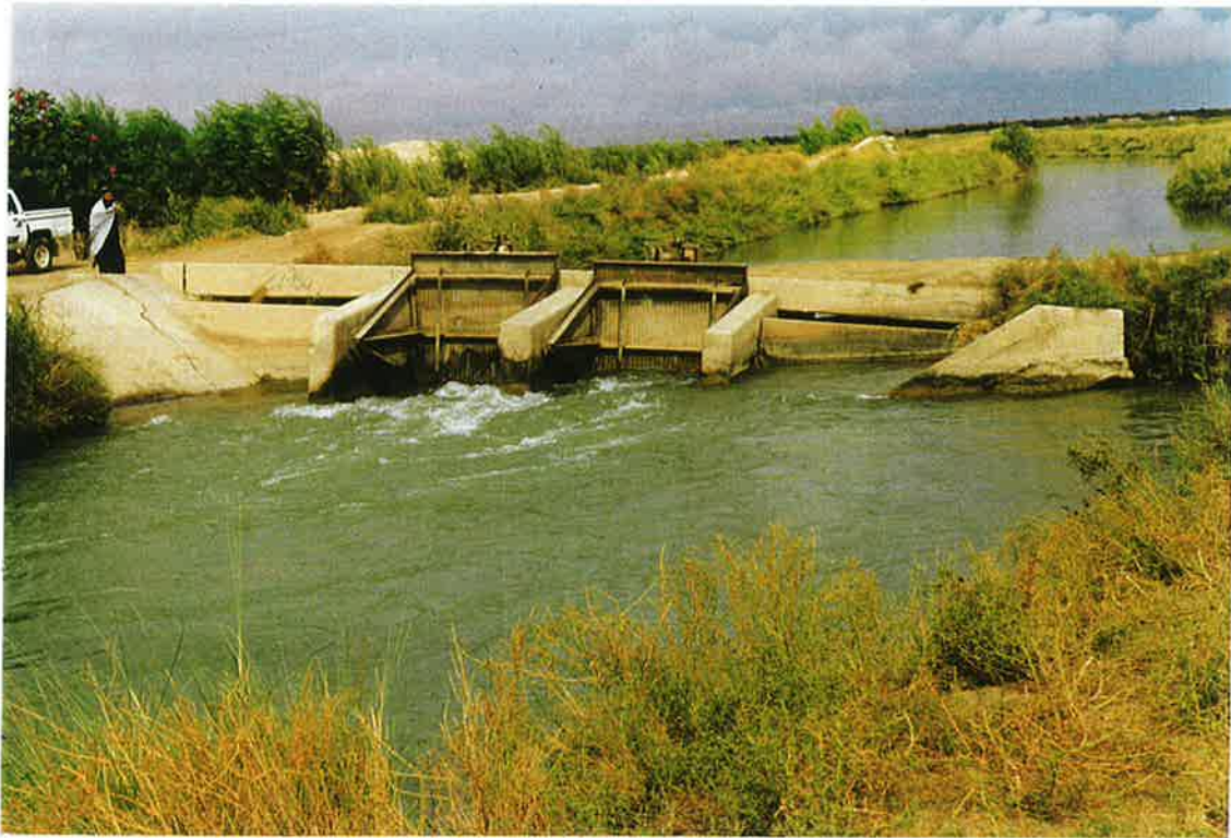
41. Damaged diversion gates on Shamalan canal at Waste way # 2. 17 Oct 97
