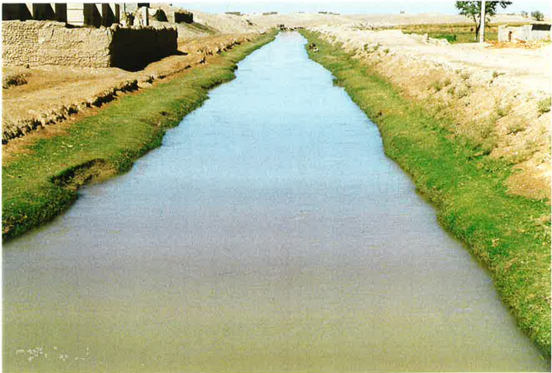
40. The S-10.7 lateral at the Lashkar Goh to Marja road in Bolan. The green grass is on silt. 20 Oct 97
