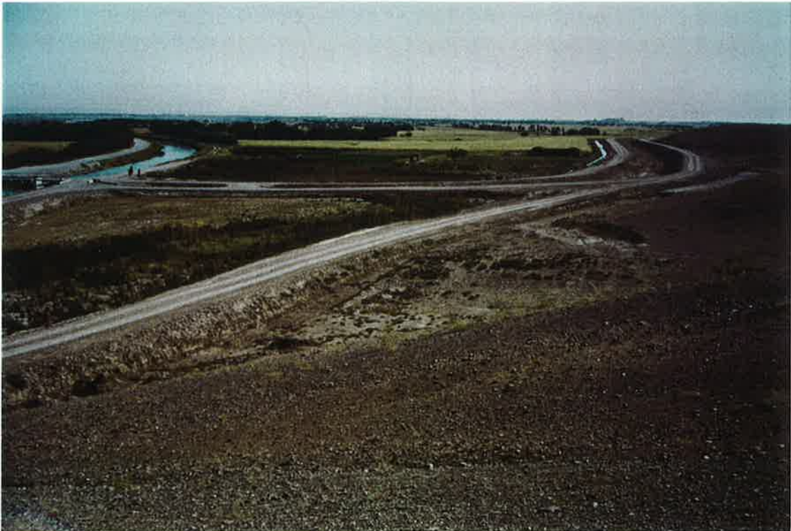
38. The S-10.7 lateral under construction. The Shamalan Canal is on the left, 1972
