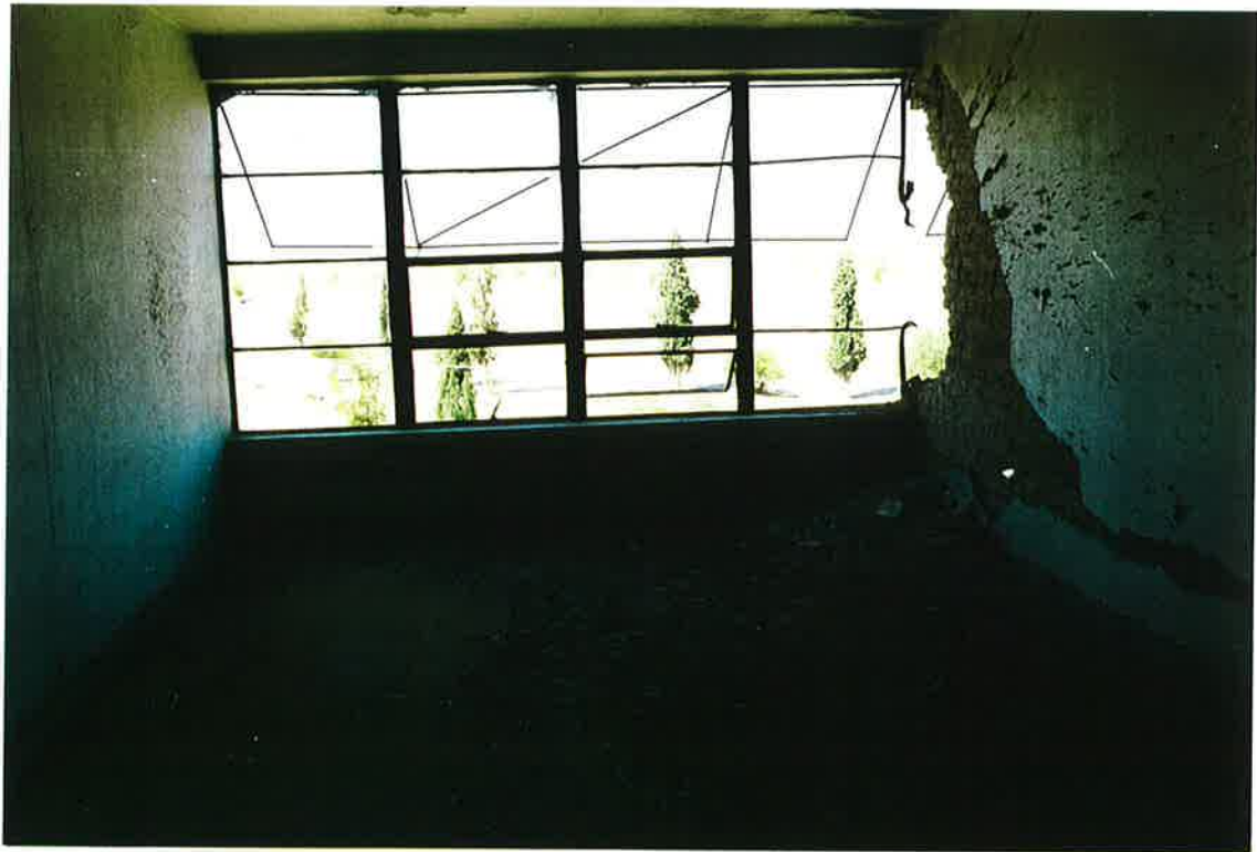
18. Damaged office in HAVA building. 20 March 97
