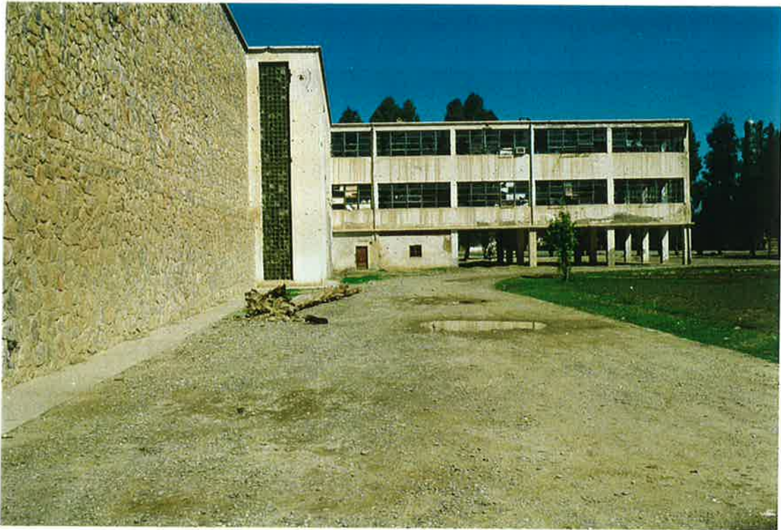
17. Engineering section wing of HAVA building. With windows blown. 20 March 97
