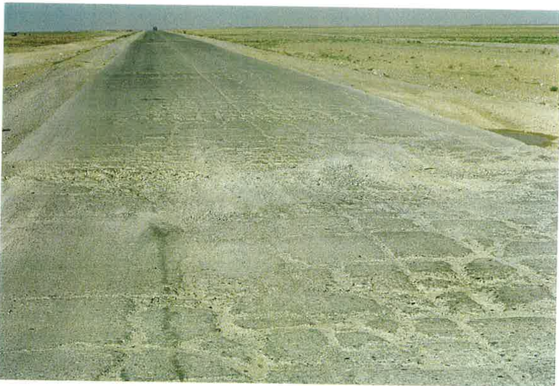
6. Kandahar to Herat highway broken road surface 23 March 97
