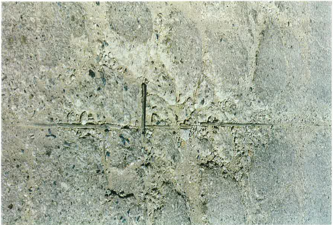
7. Kandahar to Herat highway broken road surface, close-up. 23 March 97
