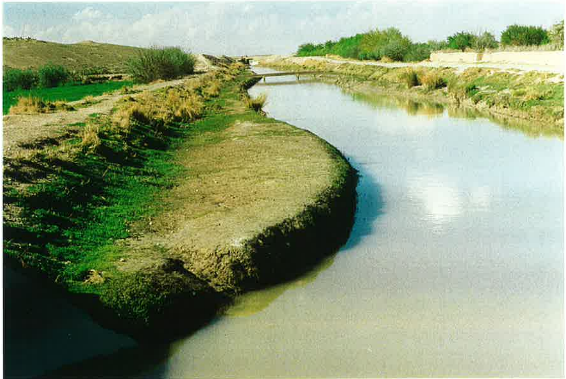
32, Shamalan Canal looking north at S-10.7 lateral intake. Note silting, center. 21 March 97
