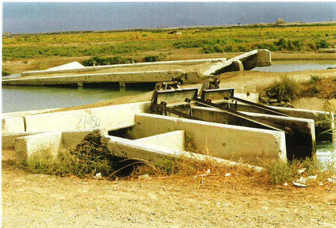
42. Damaged diversion gates on Shamalan canal at Waste way # 2. 17 Oct 97
