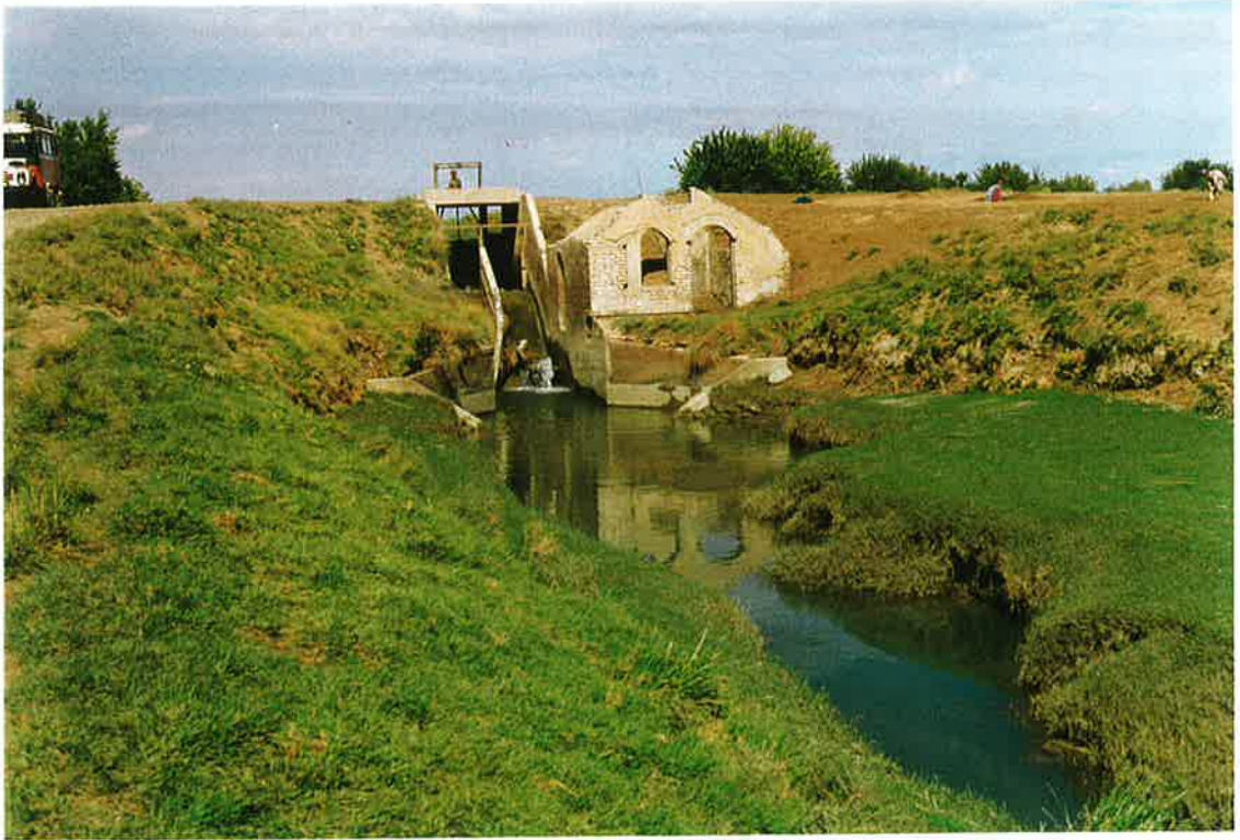
43. Silted lower Shamslan canal at drop structure and old mill. 17 Oct 97
