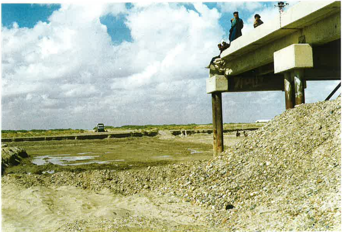
47. Washed out Darwishan Bridge approach looking west. Approach is excavated and ready for gabion fill. 17 Oct 97
