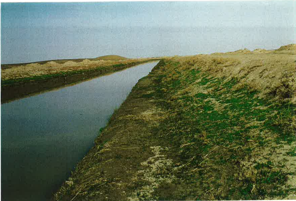
93. Silted Boghva canal near Marja from silt embankment. 22 March 97
