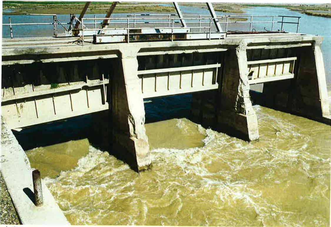
54. Diversion structure of Boghra canal intake on Helmand River. Note damaged concrete. Gates functioning. 20 March 97
