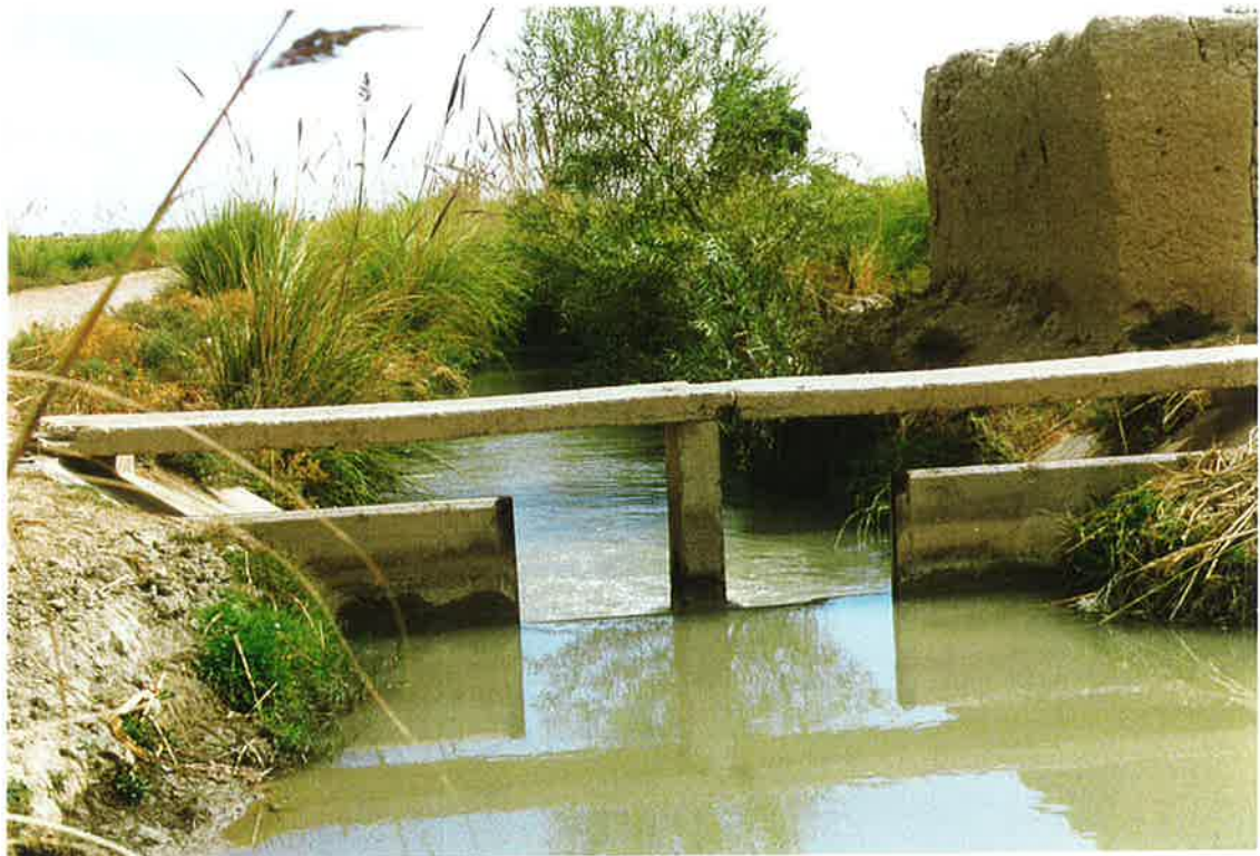
111. Central Marja over-grown channel. Gatas missing from control structure. 18 Oct 97
