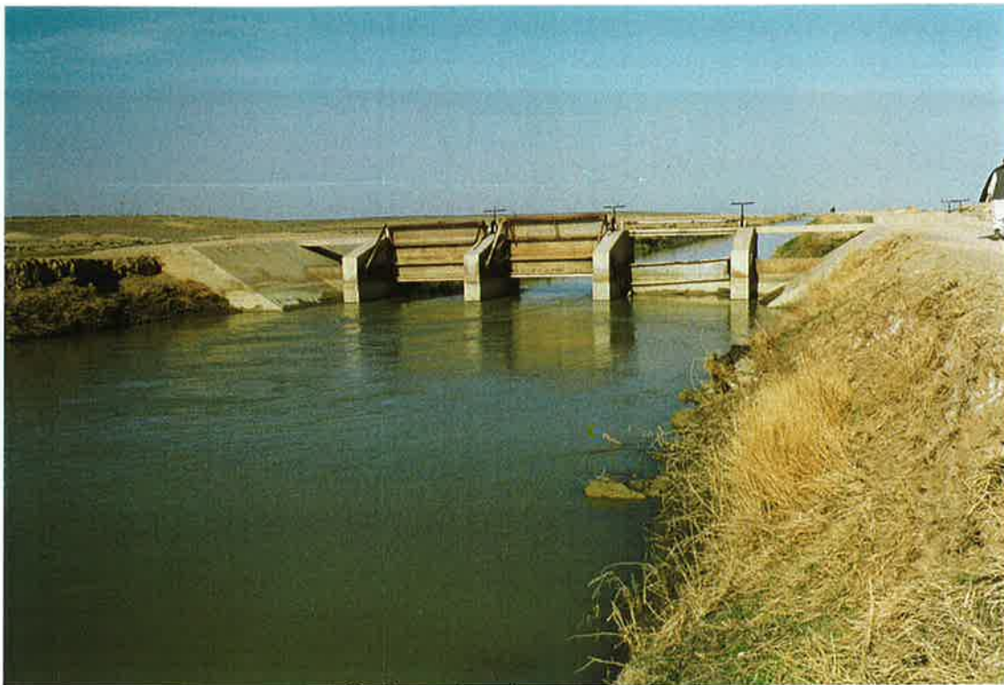
95. Control Structure on Boghra Canal at a Marja wasteway. Note washed wing on left, 22 March 97
