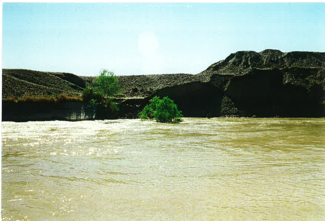
61. Washed out left wing of Boghra Canal intake structure. 20 March 97
