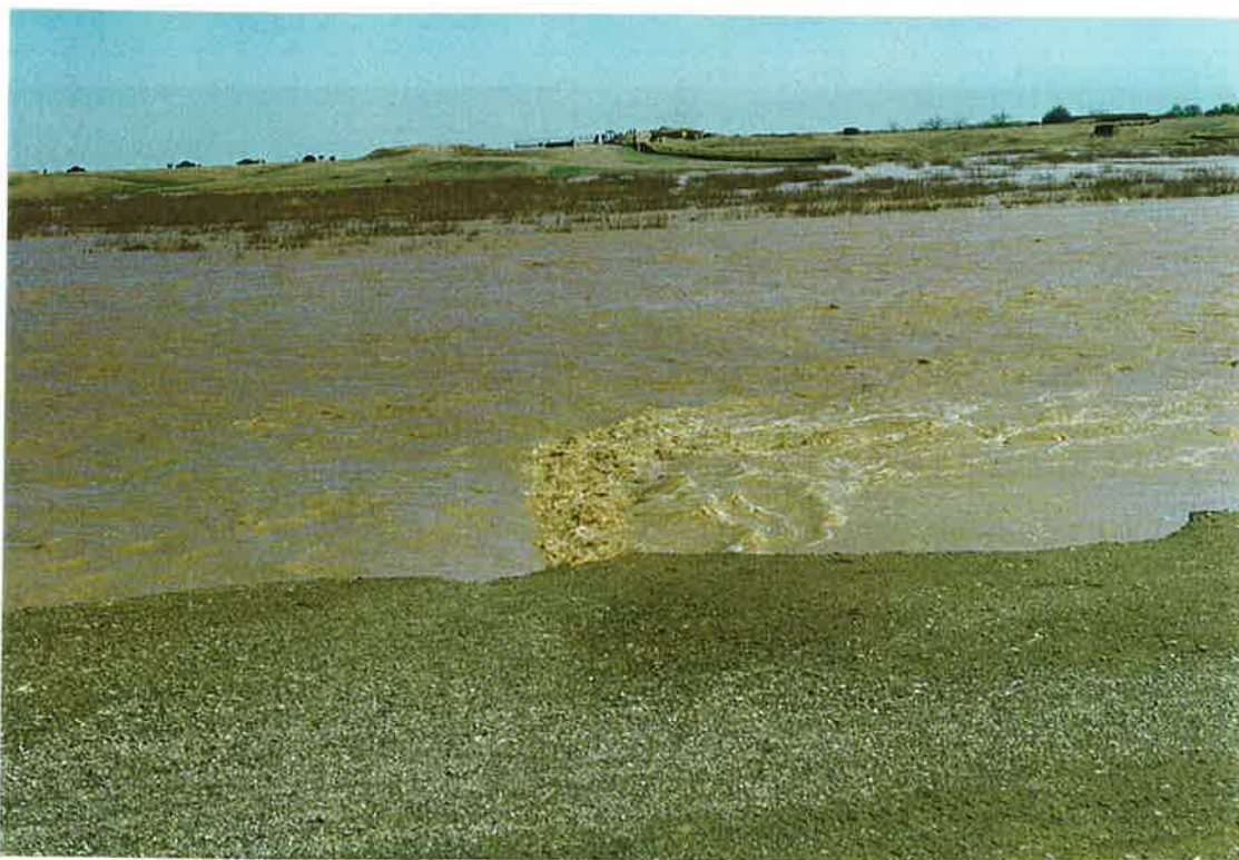
79. Lay Munda siphon being eroded out by spring flood. 18 March 97
