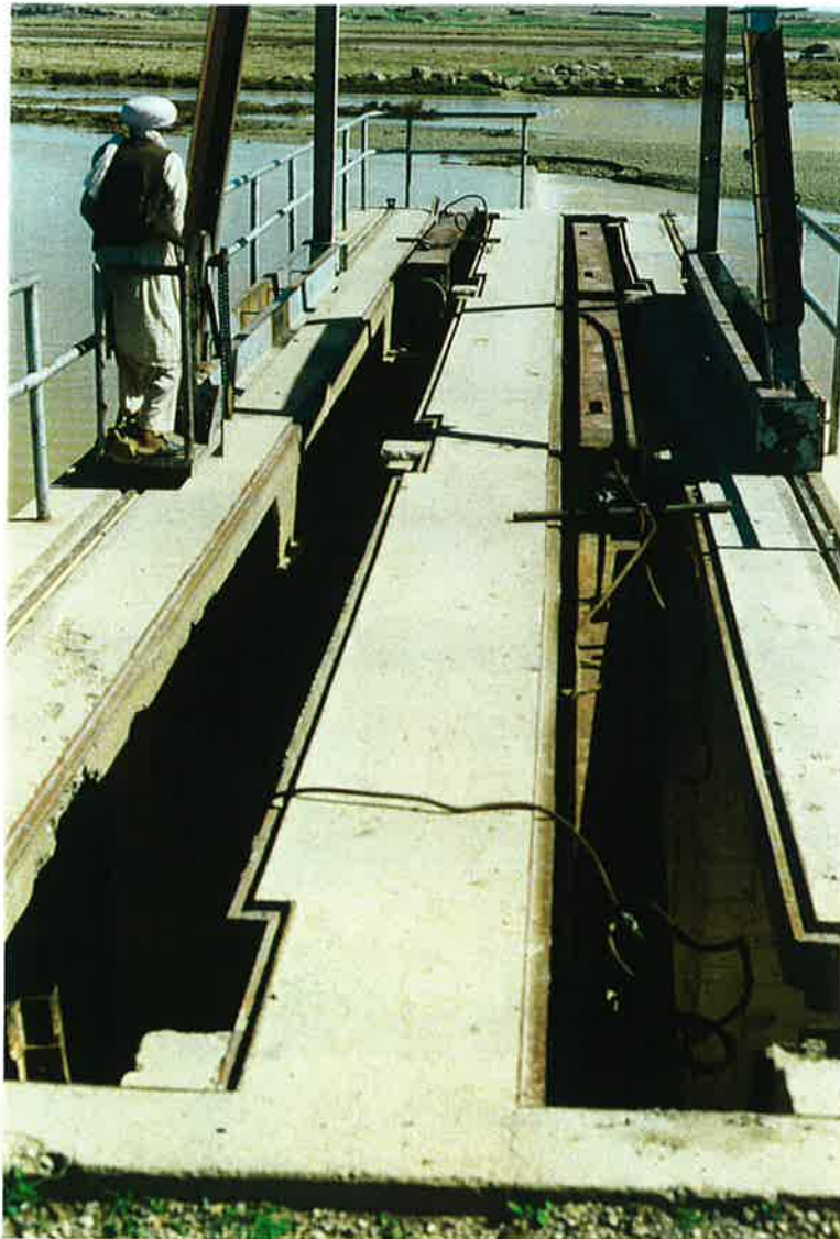
56. Gates of diversion structure of Boghra canal intake on Helmand River, 20 March 97
