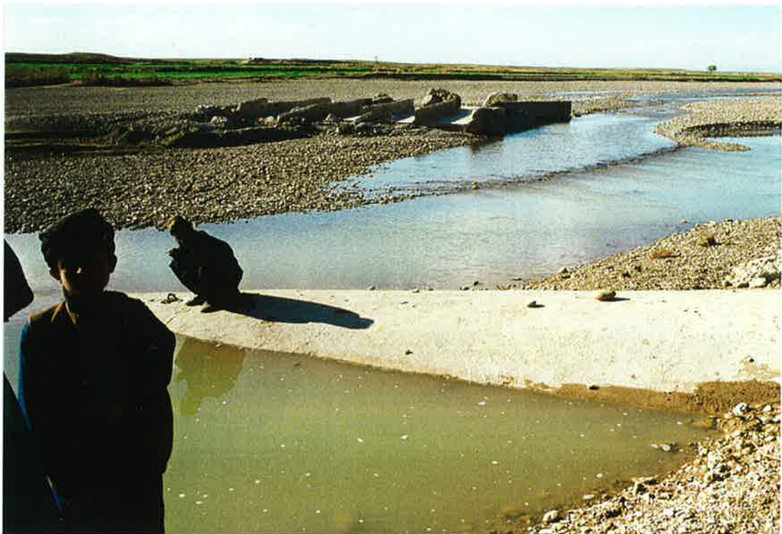
78. Exposed siphon and washed out channeling at Ab Pashak wash. In October the siphon had been re-covered by gravel/silt. 20 March 97
