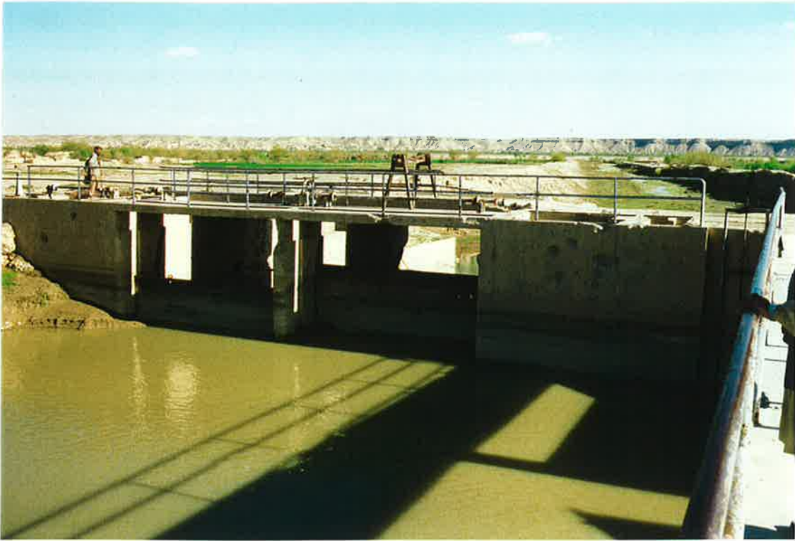
83. Waste way gates off Boghra Canal. An alternative gate lift mechanism has been made. 20 March 97 See #80-82 above.
