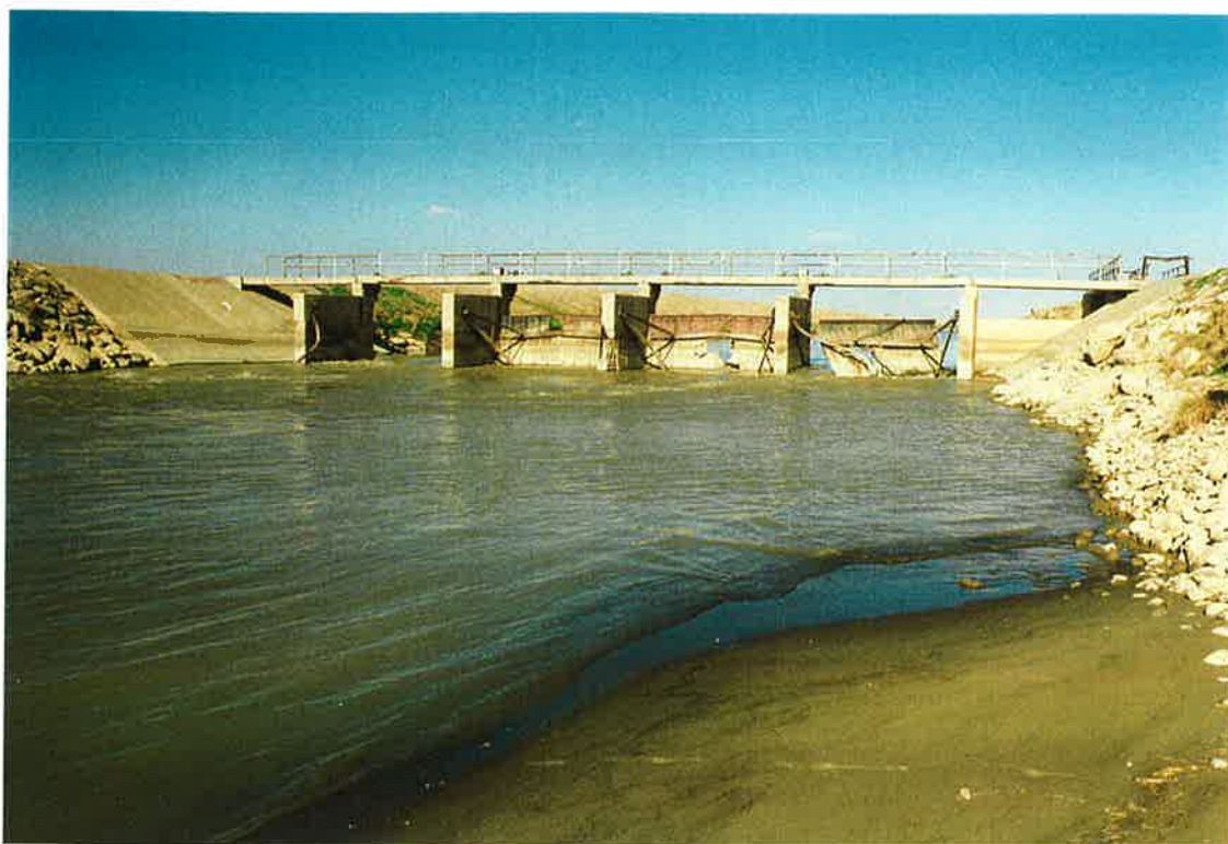
80. Control structure on Boghra canal at wasteway north of Shamalan diversion. All gates damaged and inoperable. 20 March 97
