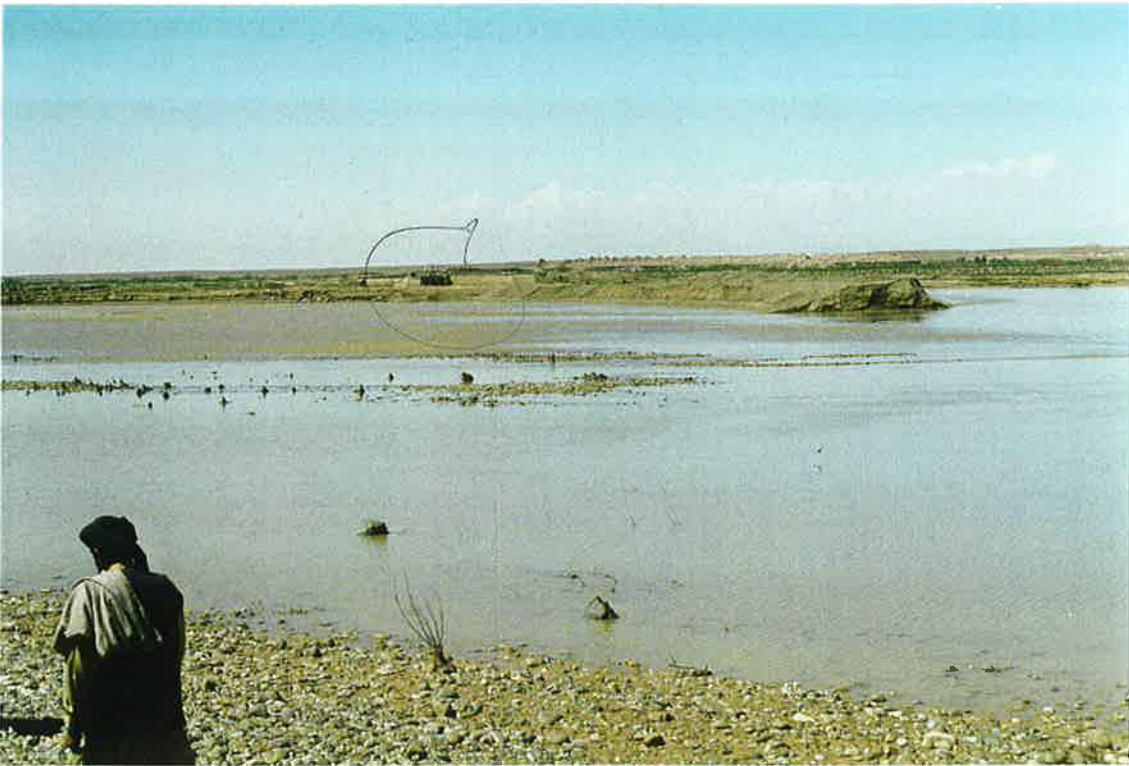
73. Recent failed river diversion dike funded by farmers from the east, The Boghra canal intake structure is left of center. 20 March 97
