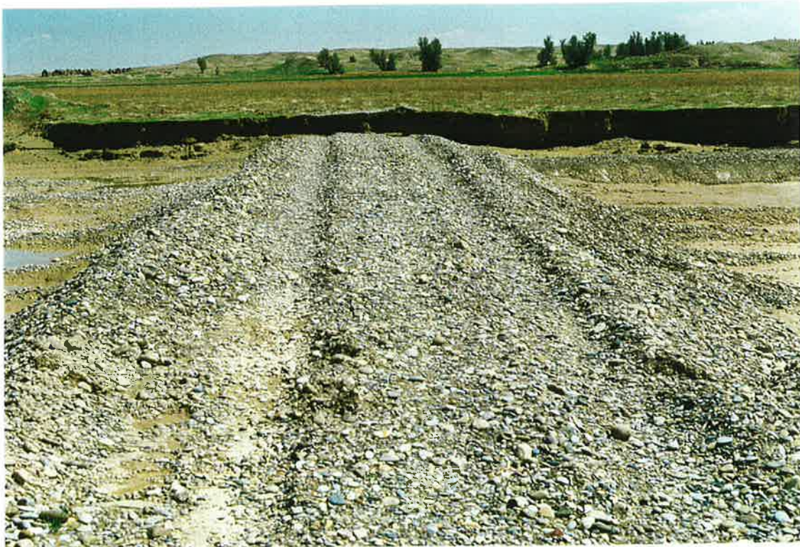
74. East end of recent failed diversion dike funded by farmers, looking east. 20 March 97
