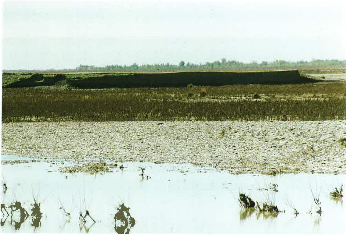
65. Old Failed MKA river diversion dike on Helmand River from north, 20 March 97
