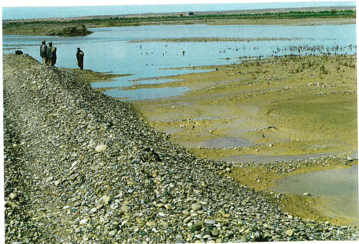
72, Failed recent attempt at river diversion dike funded by Farmers, located between the 2 MKA diversion dikes. 20 March 97
