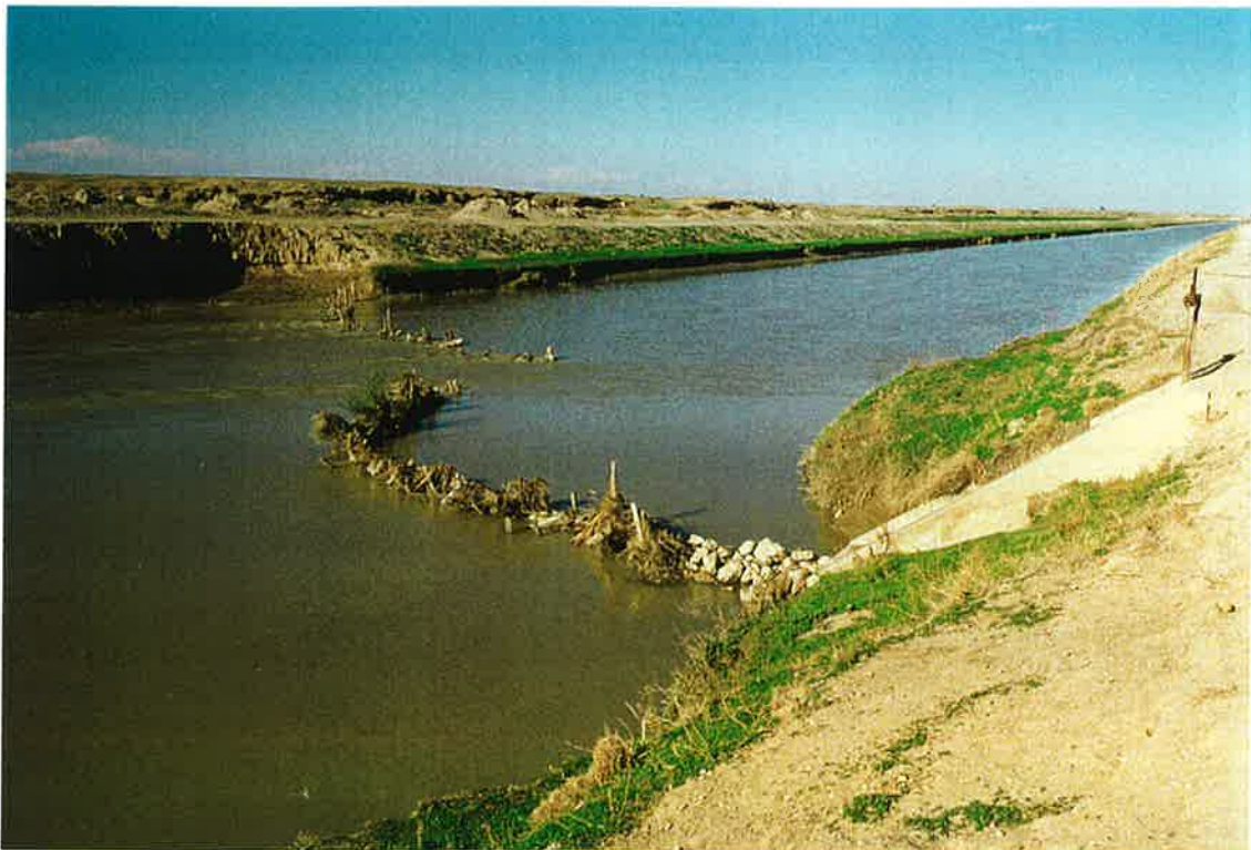
86. Farmer diversion structure on Boghra canal north of Nad-i-Ali. Note grassy silt bank on Far side.
