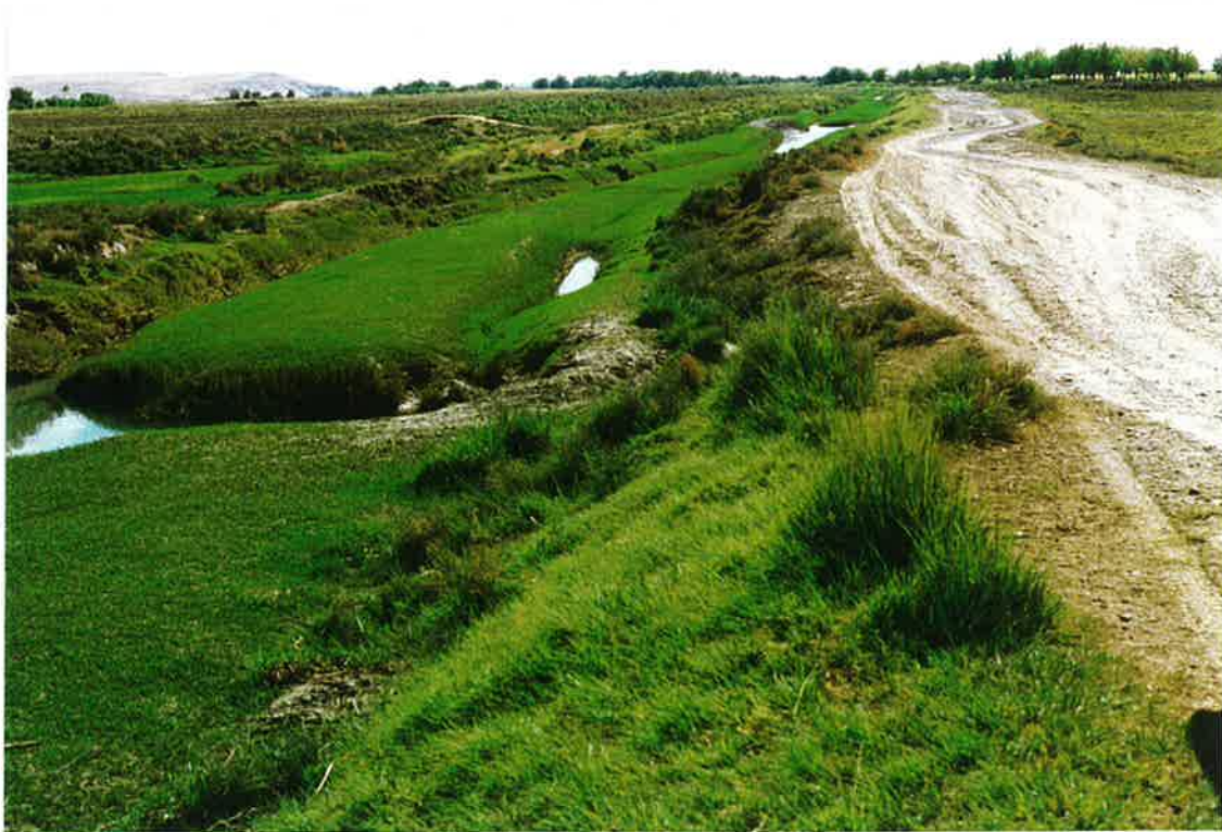
45. Silted lower Shamalan Canal in Zarist area. 17 Oct 97
