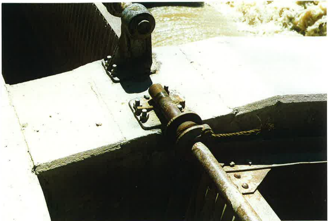
88. Gate lift mechanism part missing. See # 87 above.
