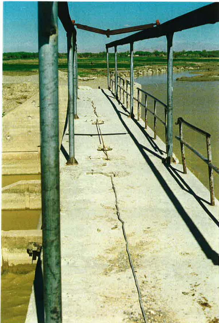
58. Baghra Canal intake structure on Helmand River with missing gates lift mechanisms. Note failed over-head lift beam. 20 March 97
