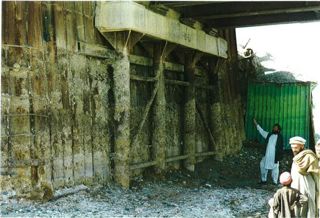
49. West end of Lashkar Gah bridge with cracked beam. Note old container being used as bridge protection from flood flows. 21 March 97
