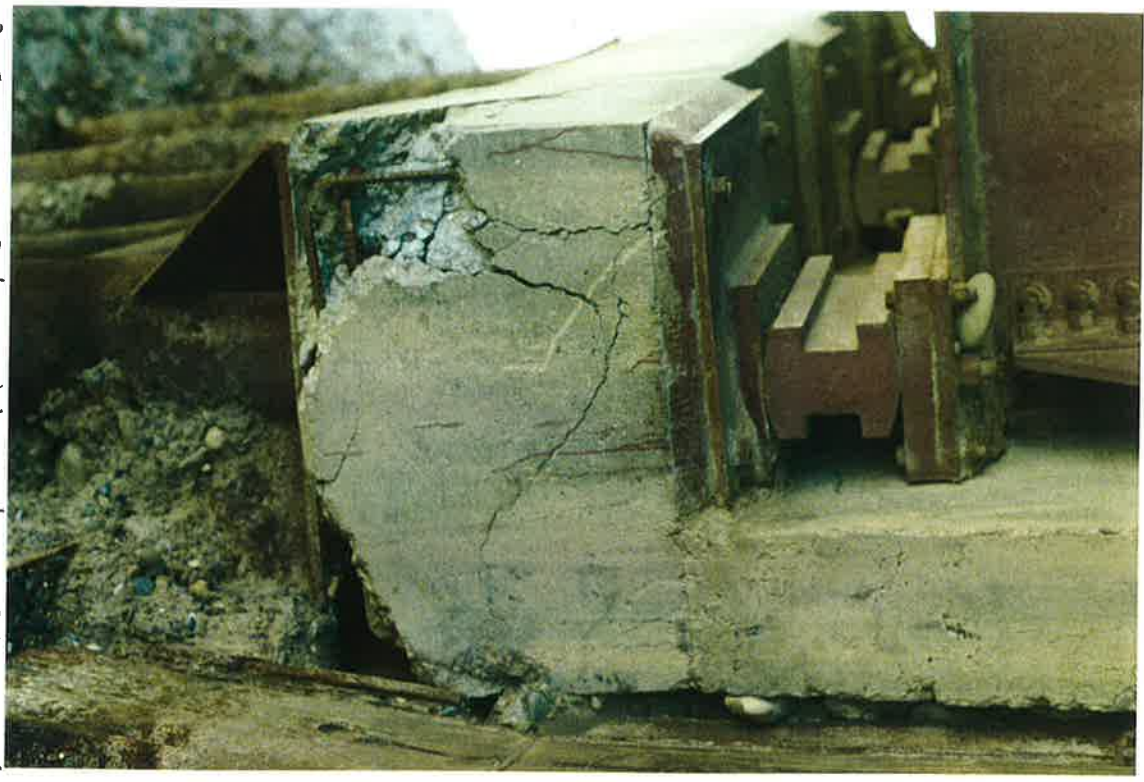
52. End view of damaged bridge beam of Loskkrabak bridge. 21 March 97
