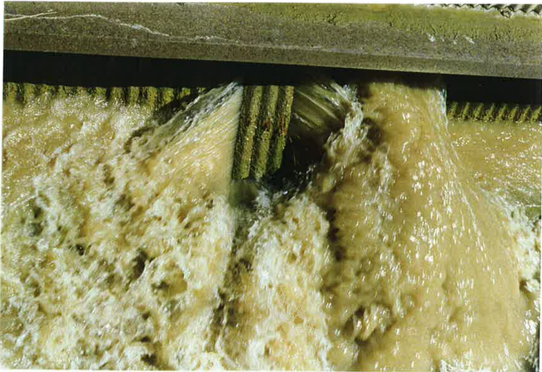
89. Damaged gate. Sec # 87-88 above. 18 March 97
