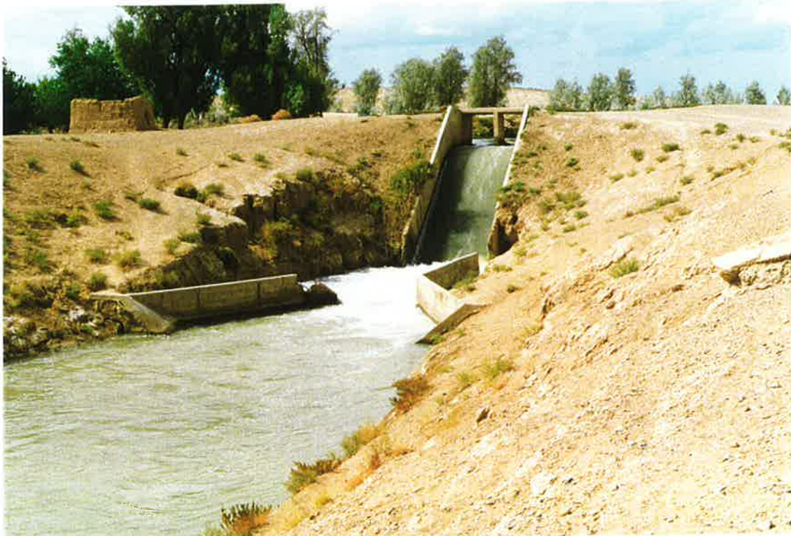
106. Damaged drop structure on Boghra canal near Marja. Note wash-out on left. 18 OCT 97
