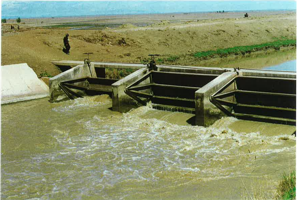
87. Control Structure on Baghra Canal at Shamalan canal intake. Gates lift mechanisms are damaged or missing
