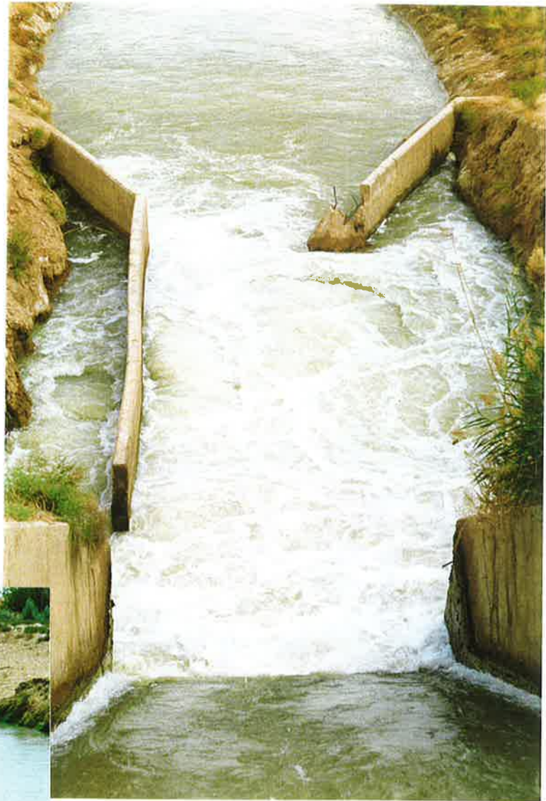
107. Damaged drop structure on Boghra Canal near Marja. See # 106 above. 18 Oct 97
