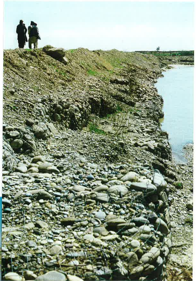
67. Close up of old failed MKA river diversion dike, down-stream (south) side with recent repairs. 20 March 97
