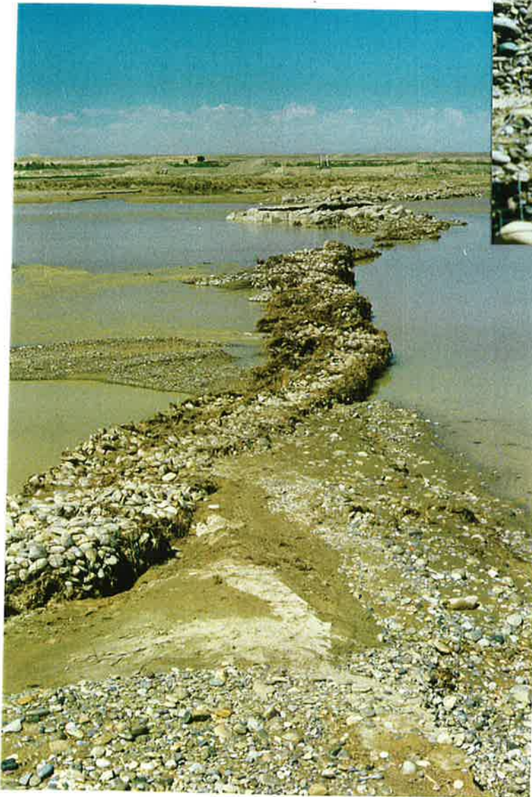
68. Close up of failed recent repairs to old failed MKA river diversion dike on Helmand River from old dike looking west.
