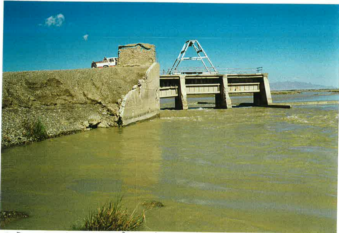
53. Diversion structure of Boghra Canal intake off the Helmand River. Note wash out on left, 20 March 97
