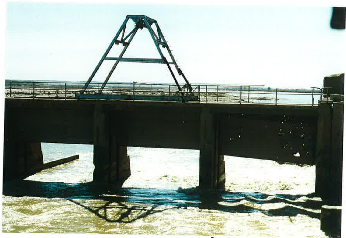
55. Diversion structure of Boghra canal intake on Helmand River from up-stream. Note damaged but functioning gate on right, 20 March 97
