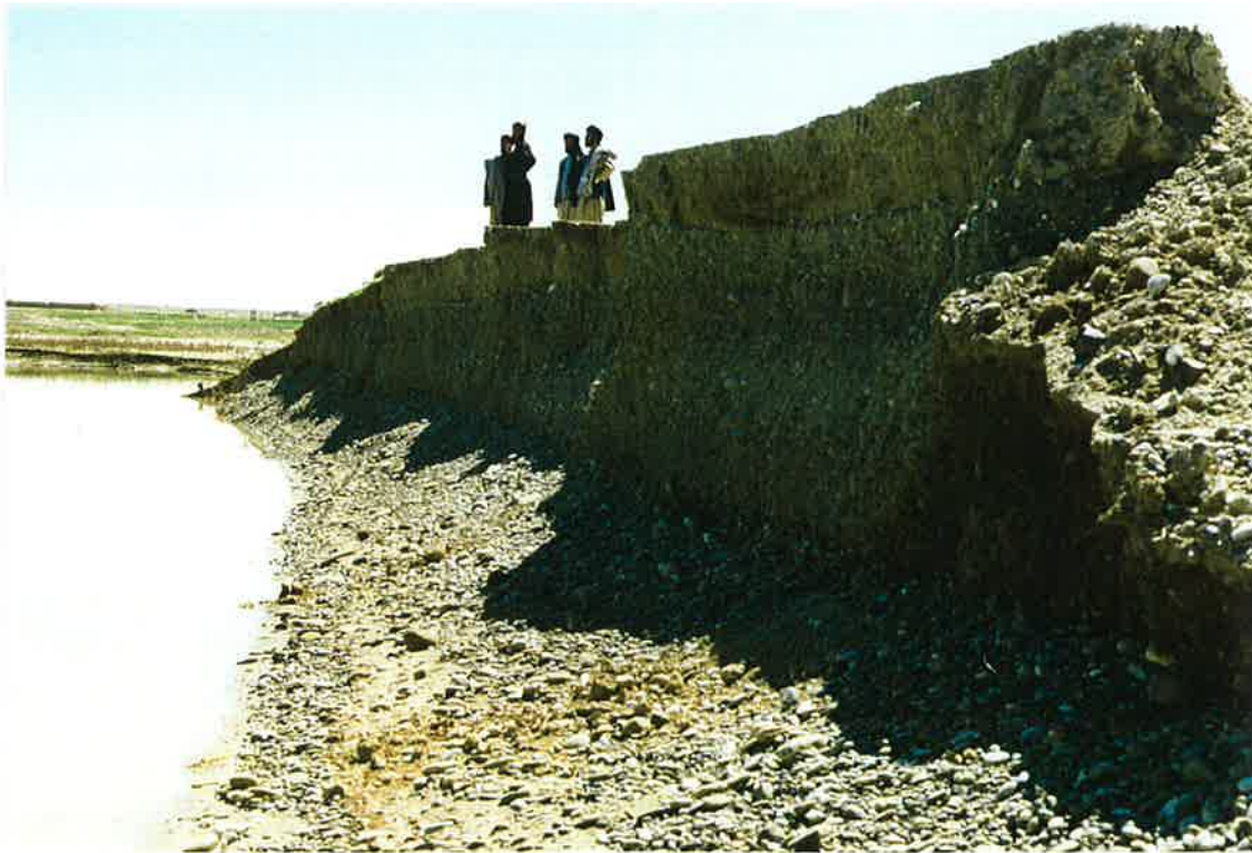
66. Close up of old failed MKA river diversion dike on Helmand River, Up stream (north) side,
