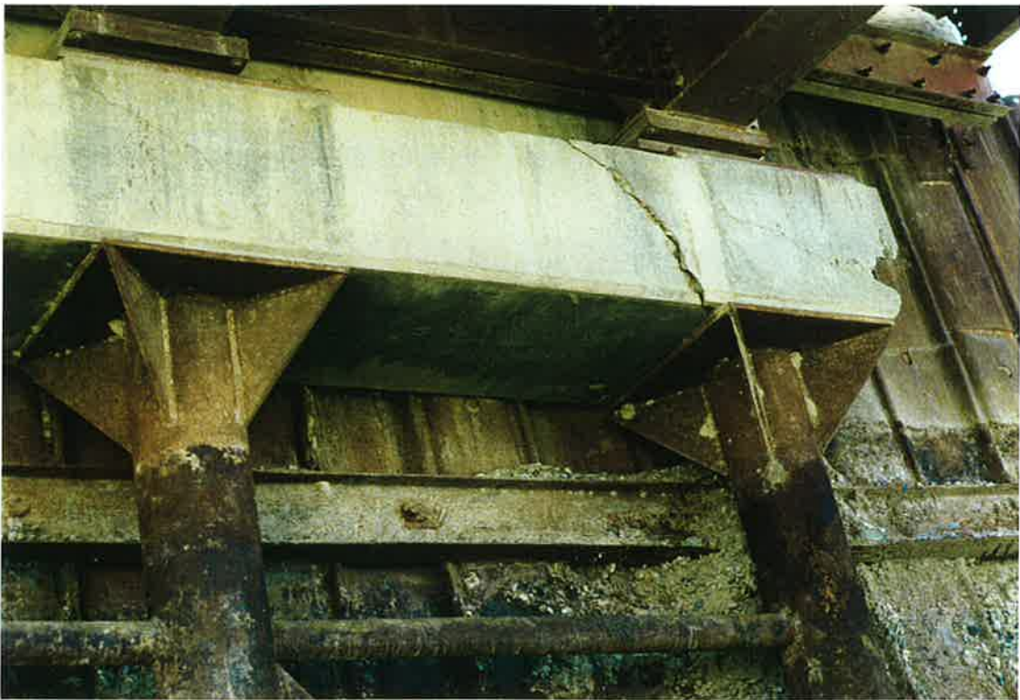
50. Close up of cracked bridge beam. 21 March 97
