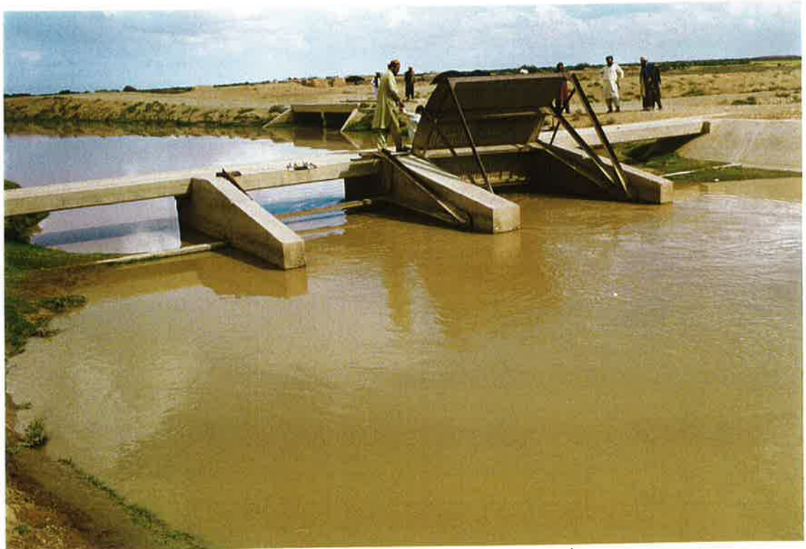
99. Control Structure at a Waste way on Baghra Canal, silted and missing gates. Near Marja. Waste way structure near top center. 18 Oct 97
