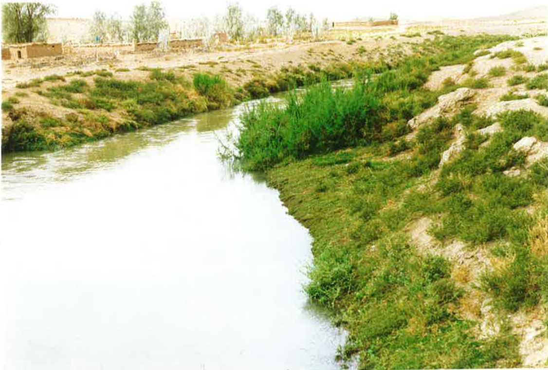
105. Silted Boghra Canal near Marja. 18 Oct 97
