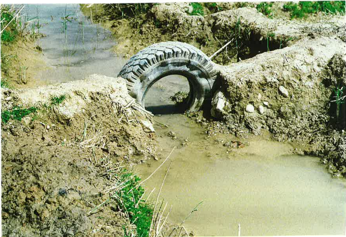
84. Farmer control structure in desert, out-of-project land near Marja. 22 March 97
